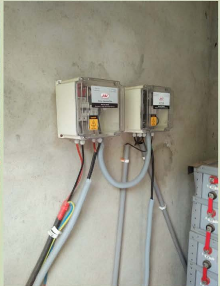
Array DC Disconnect
