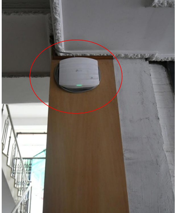
Wireless access point
