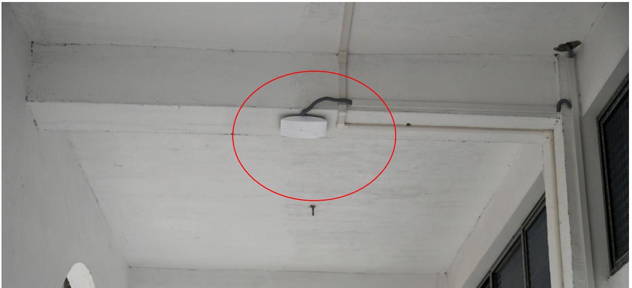
Wireless access point
